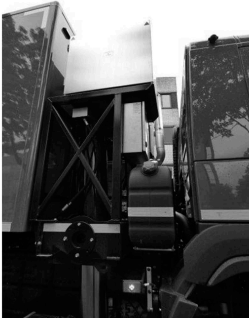
Figure 11. Batteries for the hybrid system.
