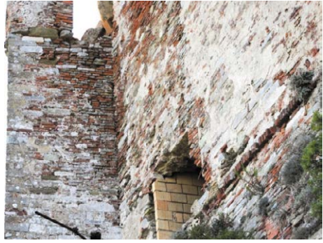
Figure 5 – In the overhanging wall the bricks are more present. Remains of the original render are visible.
