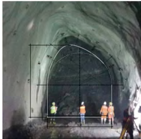
Figure 2. Initial modification of the excavation shape by Contractor to follow the failure mode (7.35 m of vertical dimension).
