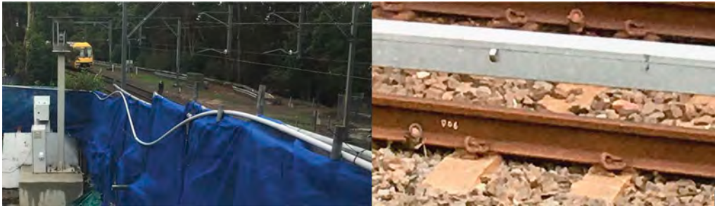
Figure 18. Automated Remote Monitoring provided Real Time Continuous Track Monitoring.
