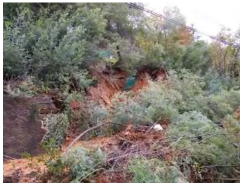
Figure 4. Landslide from ch. 2+220 to ch. 2+330 (Via Ferrania).
