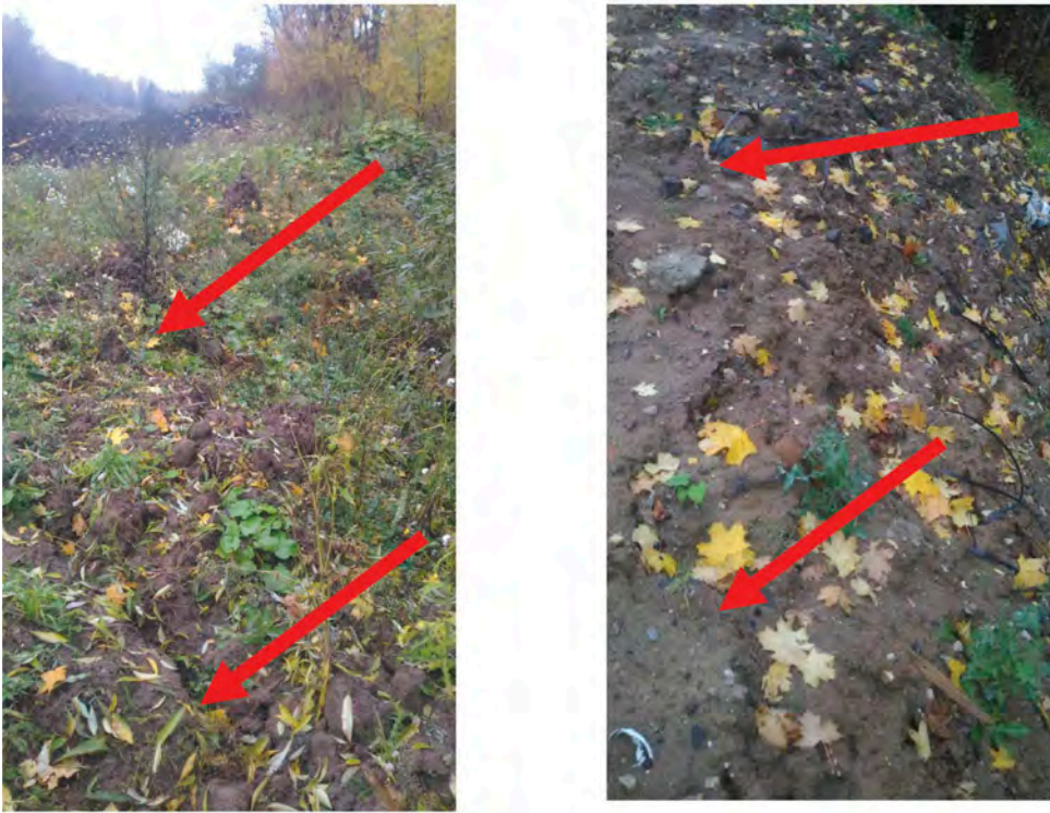
Figure 2. Cracks on the edge of the embankment.
