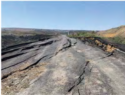
Figure 2. Damage observed on the highway.
