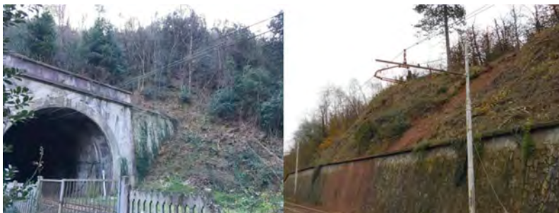
Figure 2. (On the left) Landslide from ch. 6+592 to 6+663 (Via Altare)/(On the right) Landslide from ch. 13+610 to 13+700 (Via Altare).
