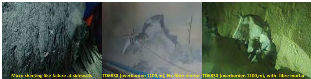
Figure 2. (a) Rock spalling at the tunnel sides (b) Rock fragments of the TBM 2 tunnel during the construction.
