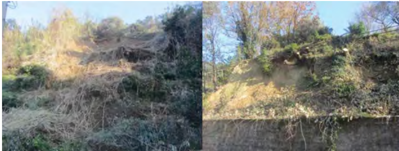
Figure 3. (On the left) Landslide from ch. 2+070 to 2+130 (Via Ferrania)/(On the right) Landslide from ch. 2+220 to ch. 2+330.
