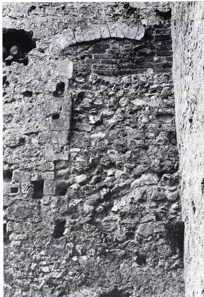
b. Blocked door leading to the first floor of the east range from the inside (pp. 51, 117)
