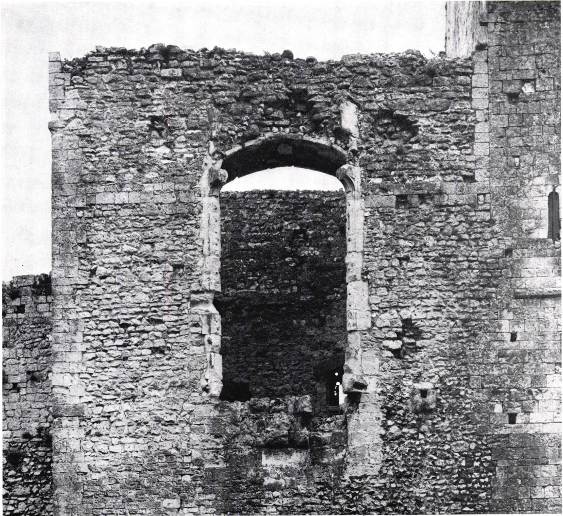
Oriel window in north forebuilding of keep (p. 84) Photograph: Department of the Environment
