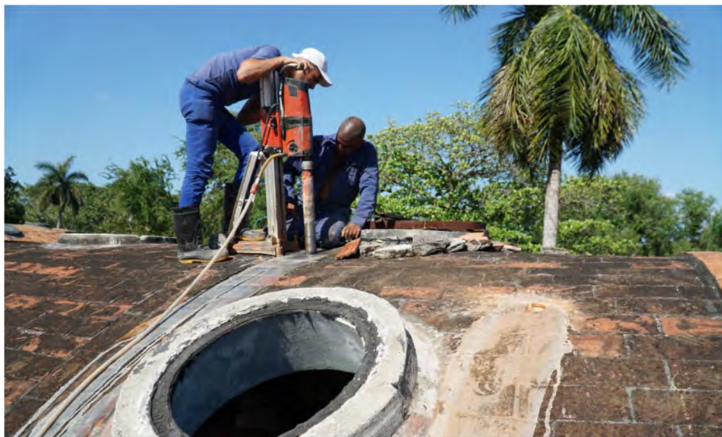
Figure 10. M. Medero Pérez (2020), Core drilling B in the top of vault of BLOCK 9 carried out by ENIA company.
