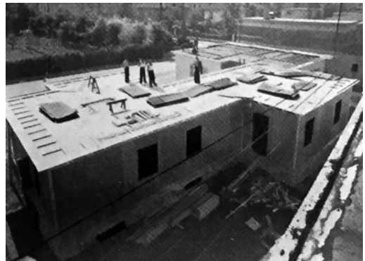
Figure 6. Houses under construction in Brescia. Completion of the roof. Source: Garda houses catalogue.
