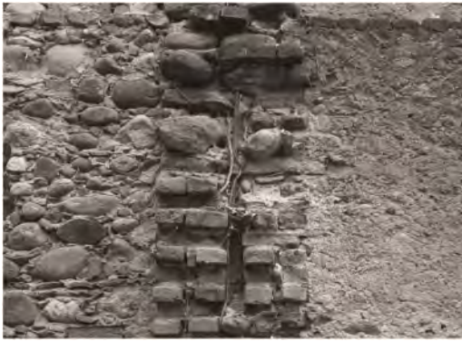
Figure 10. Montalenghe (TO), metal anchor recessed in the masonry tooting revealing the presence of a metal tie-rod in the half-width of the back transverse wall.
