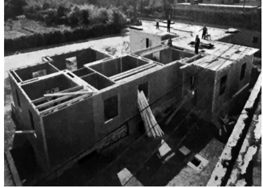
Figure 5. Houses under construction in Brescia. Roof assembly on one wing of the building. Source: Garda houses catalogue.
