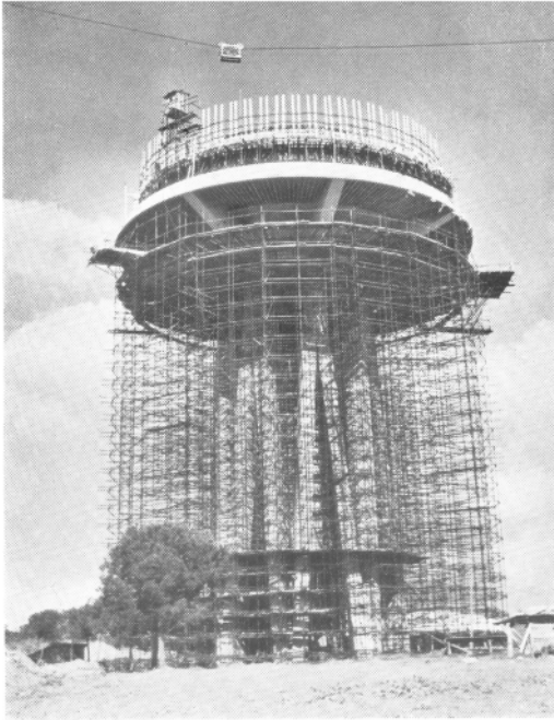
Figure 6. Roberto Colosimo Sr with Aldo Capozza and Sergio Varisco, view of the EUR Water Tower, Rome, 1957-59 the construction site was served by two antennas and a blondin .
