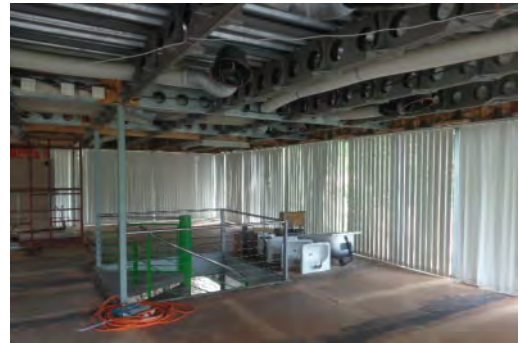
Figure 11. View of initial phases of work on the integral conservative restoration – photo Nozza C., 2015.
