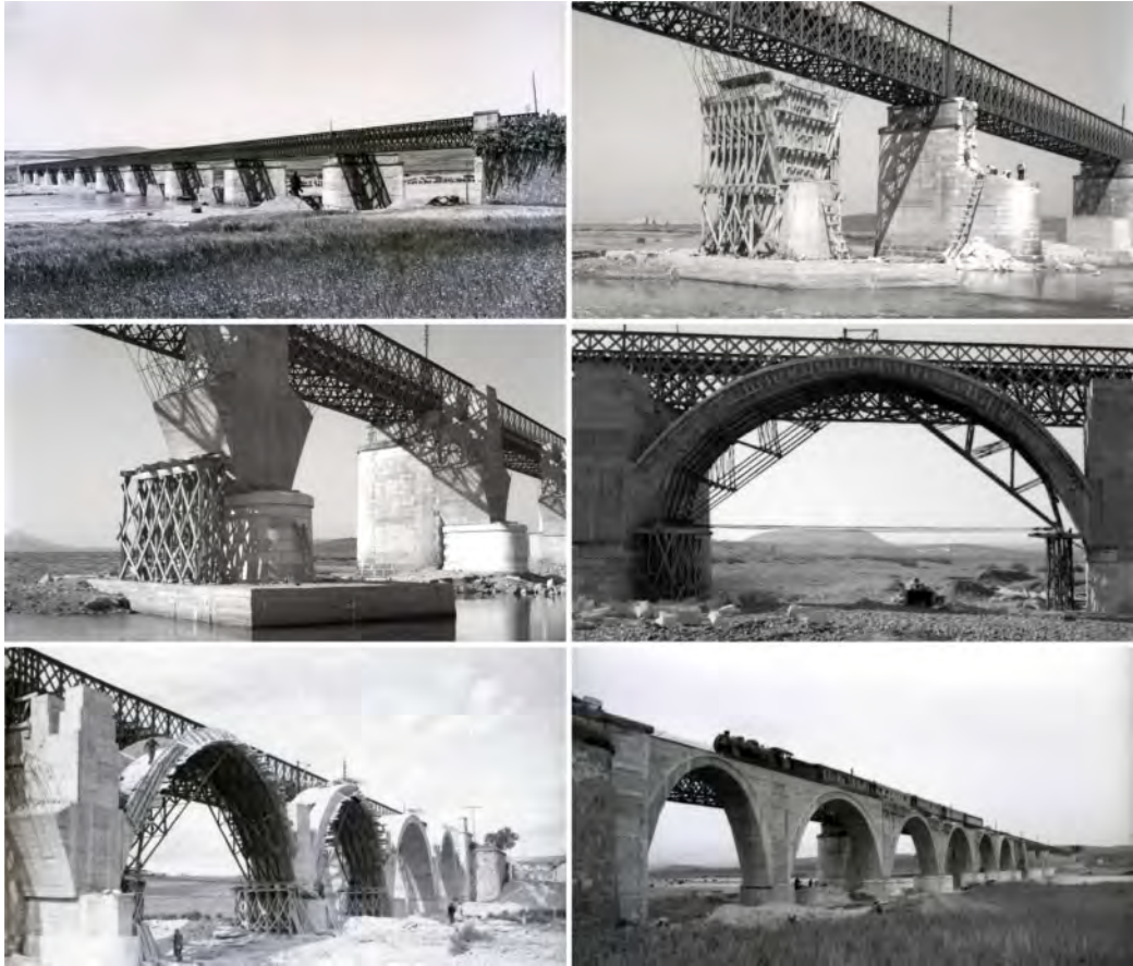
Figure 6. Zarza Bridge. Top: old bridge; execution of the new piers while former piers are being dismantled. Middle: piers already executed; centering. Bottom: groups of centerings; train on the old bridge while the new bridge is under construction. Photos by Vicente Garrido Moreno (AHF-MFM VG-IF- 2229-; VG-IF- 2244-; VG-IF- 2257-; VG-IF- 2256-; VG-IF- 2264-; VG-IF- 2288-). The collection consists of 68 photographs taken from 1954 to 28.03.1958.
