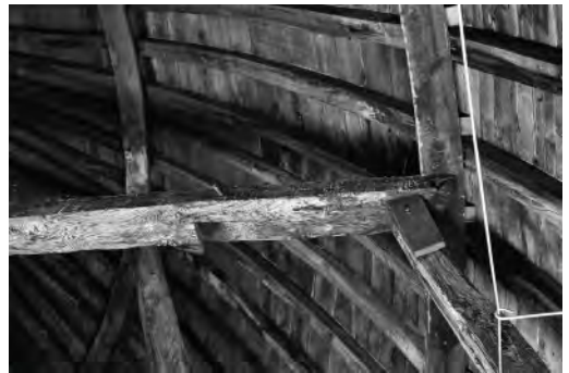
Figure 7. d02: notch visible on the bottom side of a collar-beam (photo: author).
