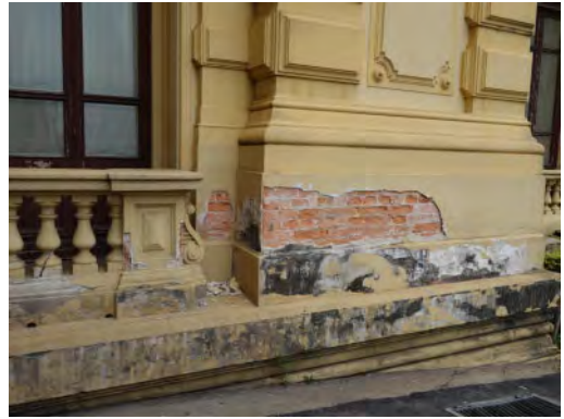
Figure 5. View of the damage identified in the external area of the building. In addition to the rising moisture stains at the base of the balustrades, there is a serious detachment of cementitious mortar and water-based paint, resulting in the exposure of the bricks without any protection or surface treatment. Source: Beatriz M. Kühn, 2019.
