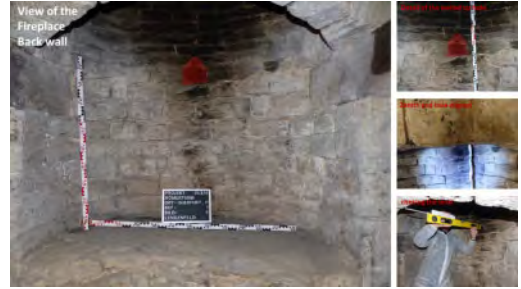
Figure 4. Photograph of the fireplace in Querfurt. Note the marked closed bearing and its position aligned with the intrados zenith of the arch.
