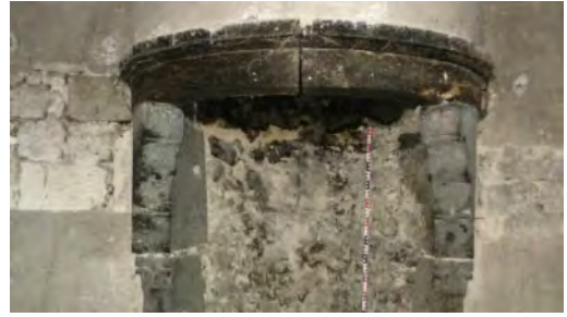
Figure 15. Detail of the wooden corbels under the mantelpiece of a chimney in Le Puy-en-Velay. (Photo by S. Schlosser).
