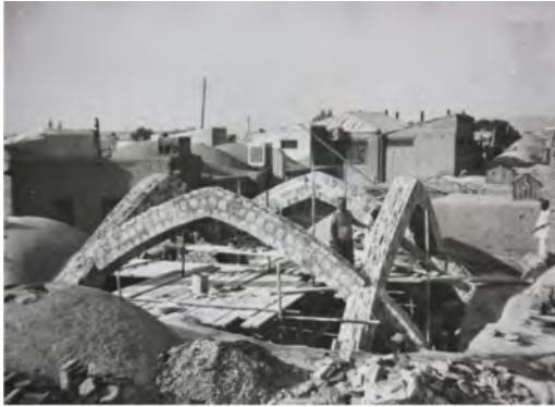
Figure 5. The Kolahduzan Dome construction. In this photo the four transverses have been built as the first phase of the construction. Farhad Tehrani archive, the photo has been taken circa 1981.
