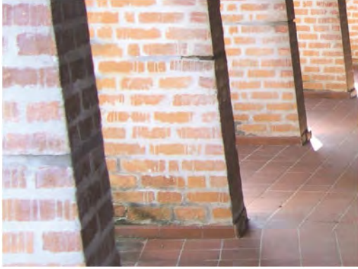
Figure 3. M. Paradiso (2003), cracks in the buttresses supporting in the entrance corridors of the School of Plastic Art.
