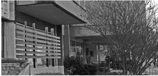
Figure 10. The missing concrete slat (to the left), digitally reconstructed in place. Image: Iva Stoyanova, 2020.
