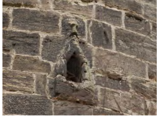
Figure 12. Detail of the chimney exiting the wall. The irregular bed joints show that this component was pre produced and fitted in.
