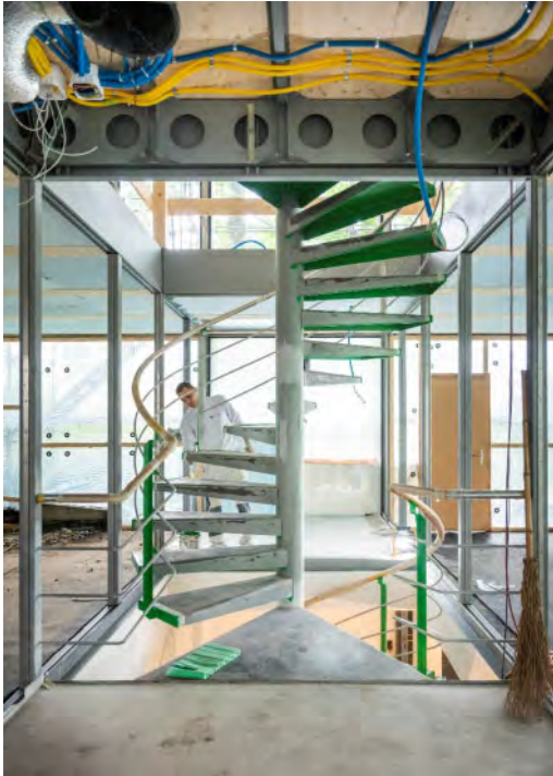
Figure 12. View of final phases of work on the integral conservative restoration – USM U. Schärer Söhne AG archive – photo Opladen S., 2019.
