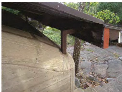
Figure 8. Ralph Erskine, villa, garage and office building in Drottningholm. Detail of the roof of the garage. The upper layer of the roof construction is completely separated from the building's structure. Photo: Elena Poma, 2020.
