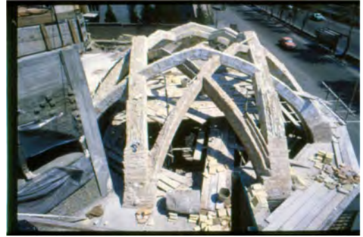
Figure 2. The construction of Masjed-i Sharif University. Farhad Tehrani archive, the photo was taken circa 1990.
