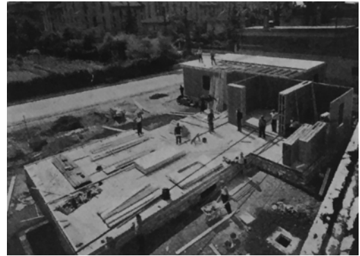
Figure 3. Houses under construction in Brescia. Realization of stone plinth and of raft. Source: Garda houses catalogue.
