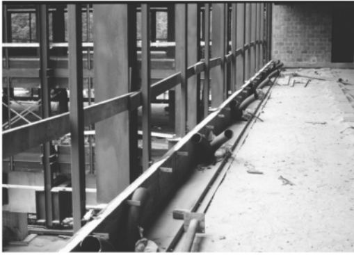
Figure 7. UPN100 profiles with welded glass beads on the building site (from the private archives of Benoît Berdoux), 1969.
