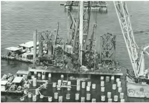
Figure 9. Lifting of a 60 m driving pile, “Elefante” platform and crane with up to 250 t lifting load (source: Simons et al. 1963).
