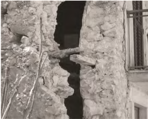
Figure 3. Villa S. Angelo (AQ), wooden radiciamenti placed in the thickness of corner walls.
