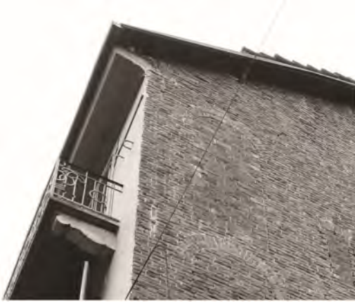
Figure 9. Turin, anchors of façade's metal radiciamenti emerging from recesses housed in the transverse wall.
