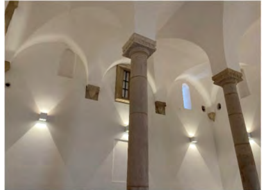
Figure 2. The visible cavities on the right corner (in relation reference to the current main entrance) above the corbel.
