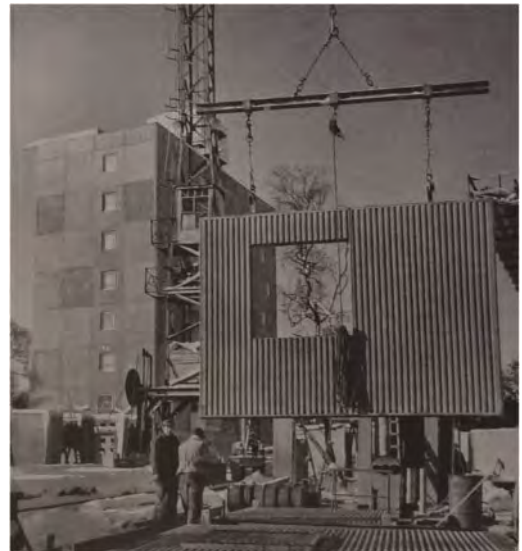
Figure 3. Construction site of Lassaskog buildings, Växjö. Positioning a precast facade panel. Photo: Sallstedts Bildbyrå / Nordiska museet.
