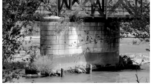
Figure 4. Cruet Bridge: a pier and its upper rubble masonry sustained by pneumatic foundations (Decker 2020).
