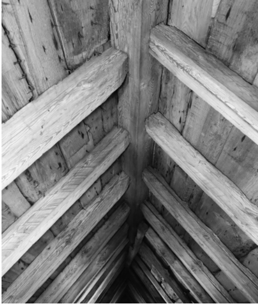
Figure 5. Detail of the ridge purlin in the roof of Valtorp Church. Note the “sprätthuggning” on the rafters. Photo. M. Hallgren.
