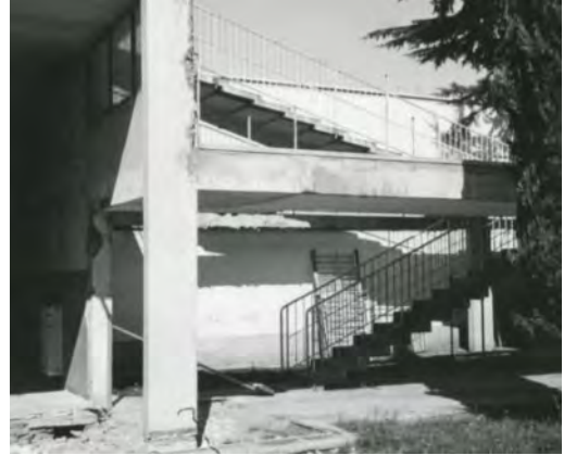
Figure 8. Worksite during the second restoration project: the reinforced concrete structure with the stairs giving access to the solarium. There is visible non-structural cracking, trickling and staining in the plastering surfaces; spalling of the concrete cover in the pillar’s corner; evidence of previous repairs. (AT ca.late 1980s).
