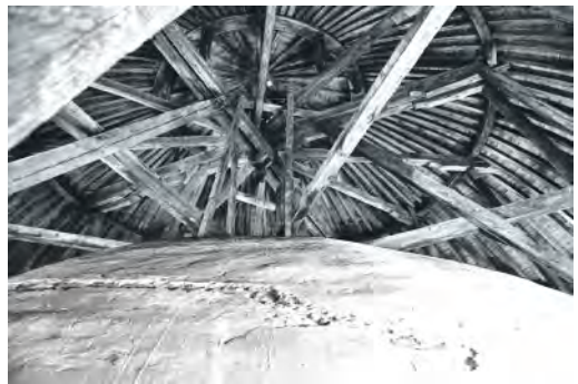
Figure 2. d02. Interior of the attic with the masonry vault and the wooden superstructure (photo: author).
