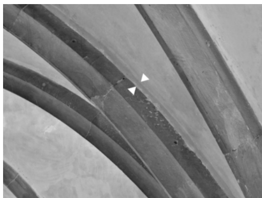
Figure 2. Klingental Monastery, Basel. Detail of the vault, the white marks indicating the gap between the rib and the intrados (photo: author).
