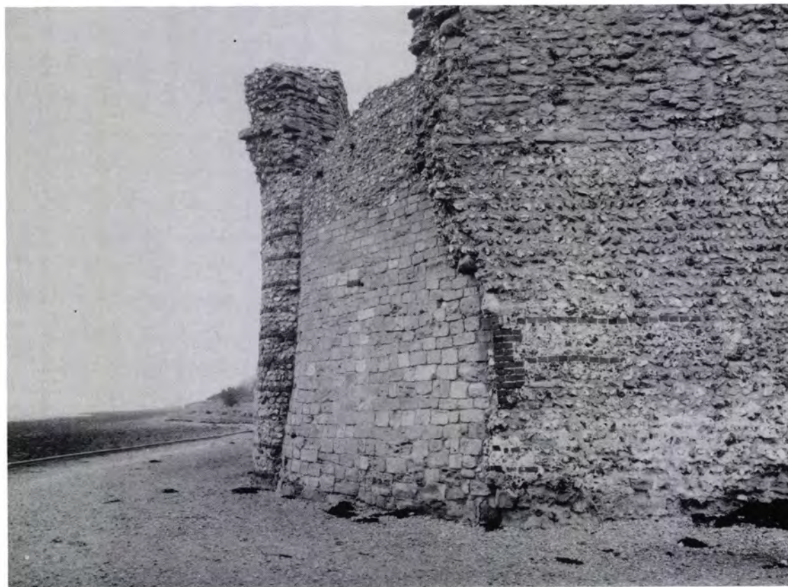
b. Bastion on the south curtain wall showing different styles of post medieval patching with Roman work above.
