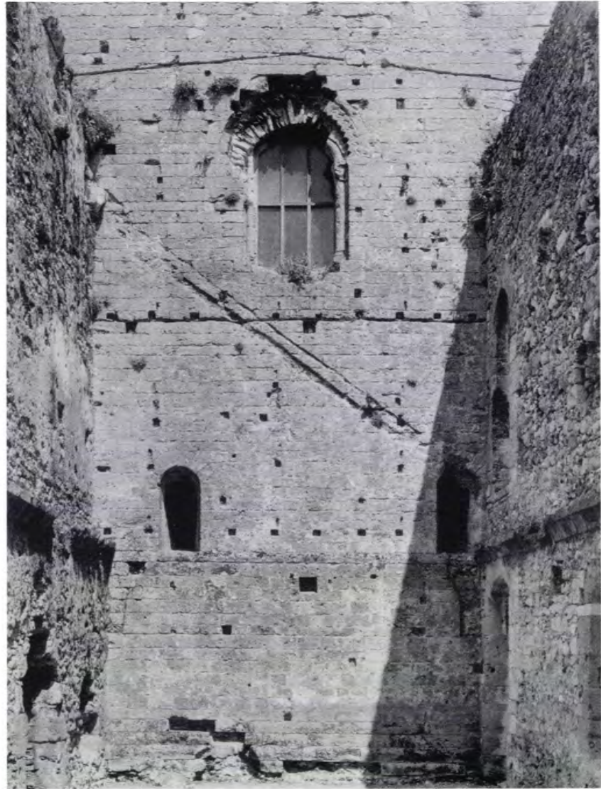
b. South wall of the keep from within the west range showing a roof line (the lower roof line) of post medieval date.
