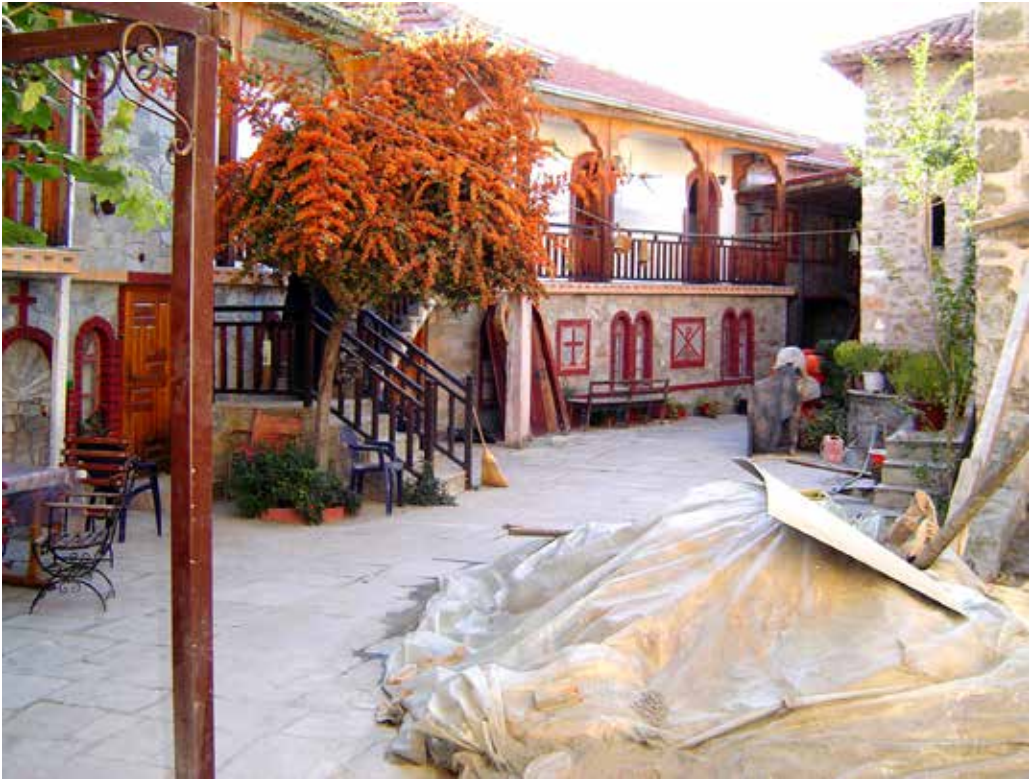
Figure 45: The Varlaam monastery: internal view C (source: author's photo). This is the space (to the left of the door: see figure 43) used by the monastic community. Construction works are in progress. Due to the fact that the visitors occupy the largest part of the monastery, including the katholicon (see figure 44), the monastic communities have to create new space within the monastery (as indicated by the construction works).
