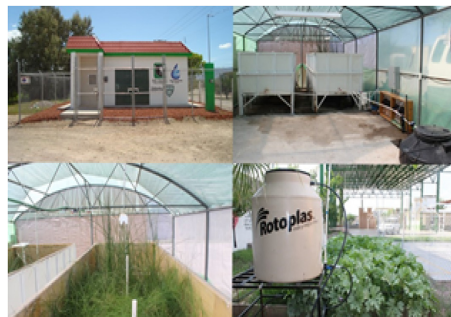
Figure 2. Pilot system implemented to remove arsenic from reject water of reverse osmosis system through constructed wetlands in Julimes, Chihuahua Mexico.
