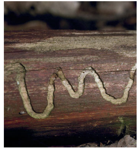
12.55 Beetle galleries in the wood of a post.
