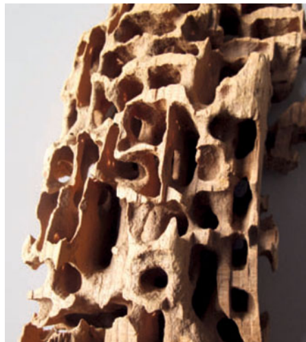
12.76 Galleries of carpenter ants.
