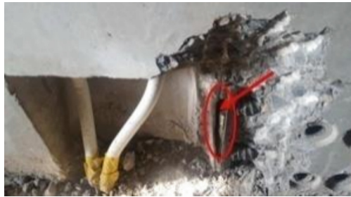
Fig. 1. The reinforcement sleeve is not full grouting
