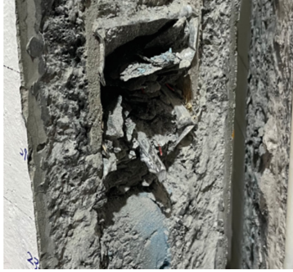
Fig. 11. The dowel was cut off in SKJ 1 specimen
