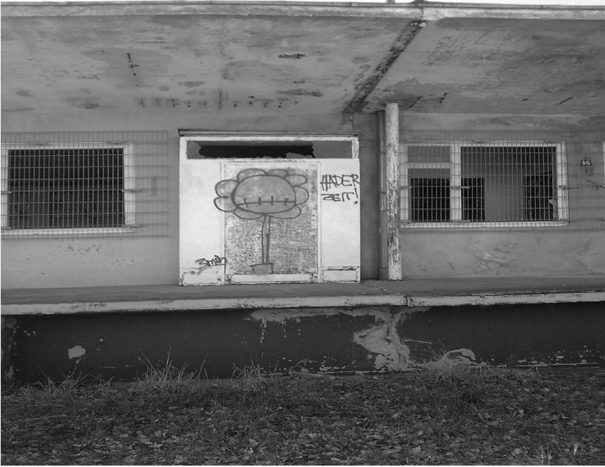
1.5 Ruins of border truck stop, Wyler, Germany, showing graffiti
