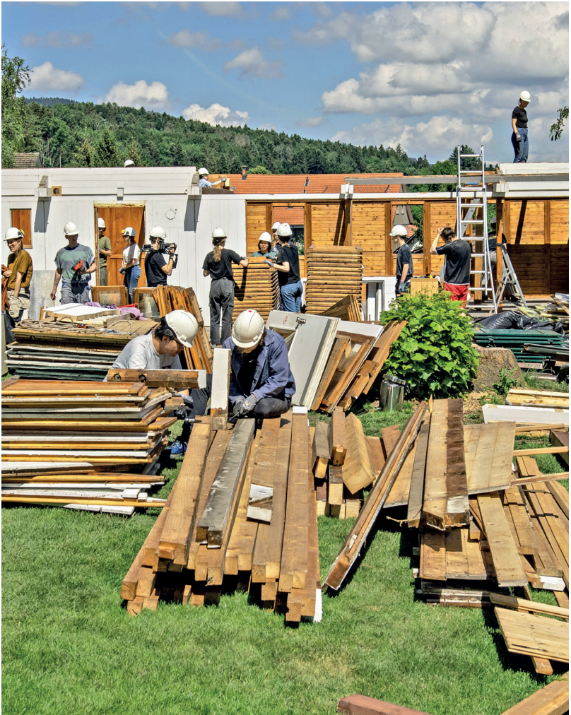
Demolition materials are sorted by hand and with the help of laser scanners and robots, then marked with QR codes and recorded in a database.
