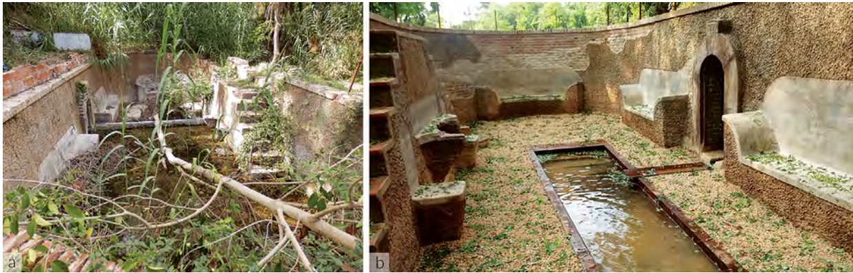
Figure 3.6a and b The Can Moritz spring, Rubí, a) before and b) after the final renovation (Source: Mireia Gascon)
