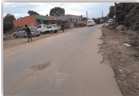
Figure 3. Bangwe to St.Patricks Road with poor shoulders and without a drainage system.
