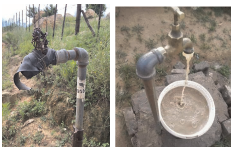
Figure 5. Poorly maintained water infrastructure.
