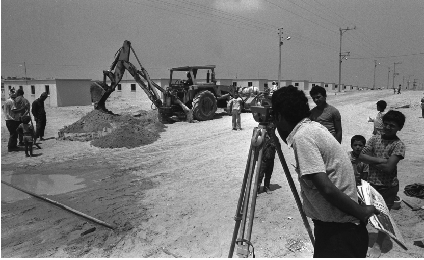
Figure 6. PWD during the construction works at Sheikh Radwan Neighbourhood, 1976 (National Photography Collection, photo by Moshe Milner).
