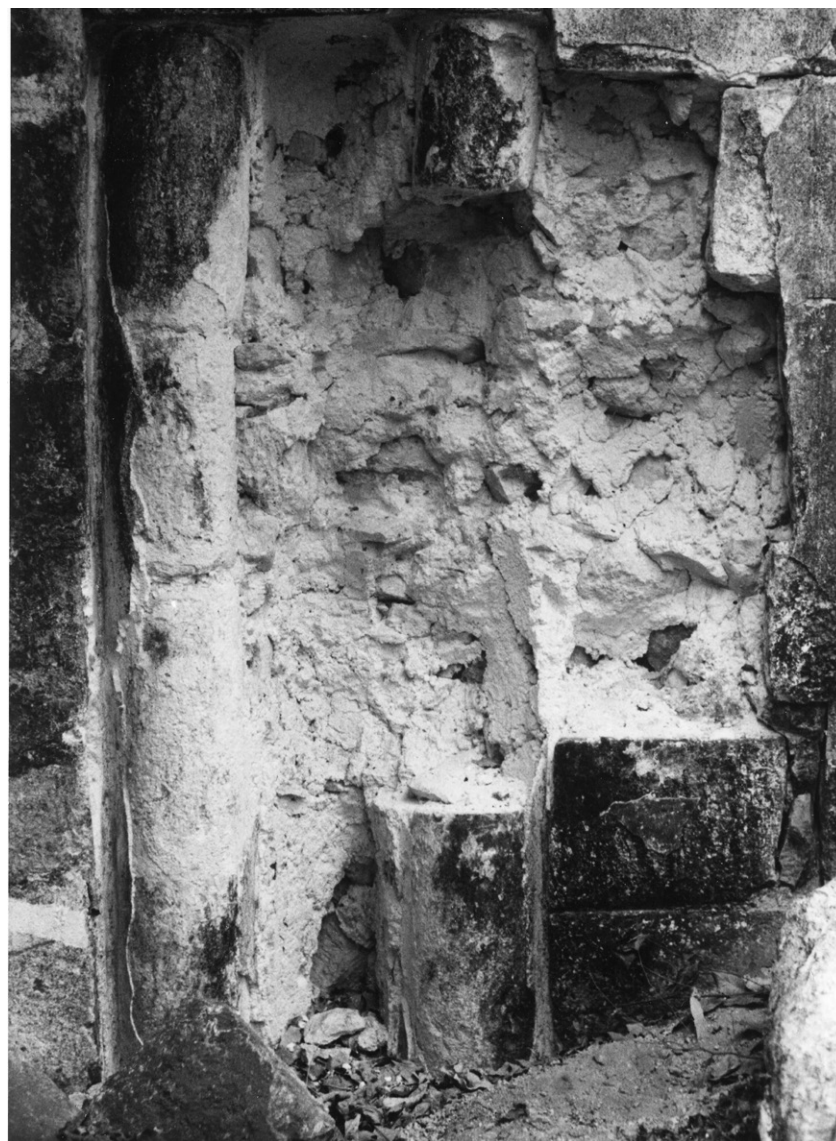
Fig. 127 The situation after the looting of the western sculpted half column of Room 1 was a serious static problem for the Palace. Photograph: K. H. Mayer 1986
