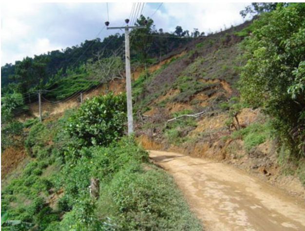
Fig. 11 Immediate upper slope (slope section above the road) de-stabilization, Kalawana, Ratnapura, 2003
