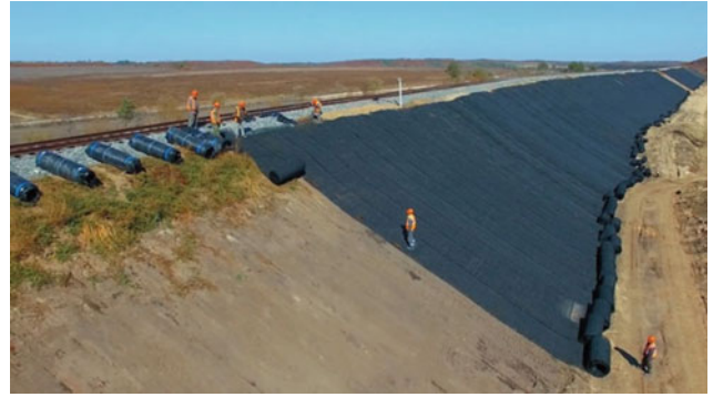
Fig. A.2 Geosynthetics used to stabilize a slope by interacting with vegetation root structures
