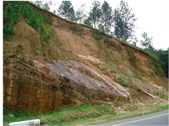
Fig. 12 Failure observation of a road side slope cut section which was constructed at 0.5 to 3.5 m high without any retaining structures
