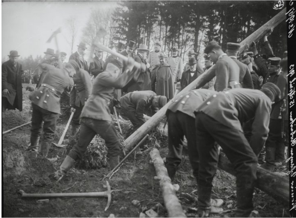
Figure 28.4. Saalburg 1913. Earthwork A. Preparing the posts and cleaning the building plot of bushes. Saalburg Archives Neg. No. SbA_SR02.002.
