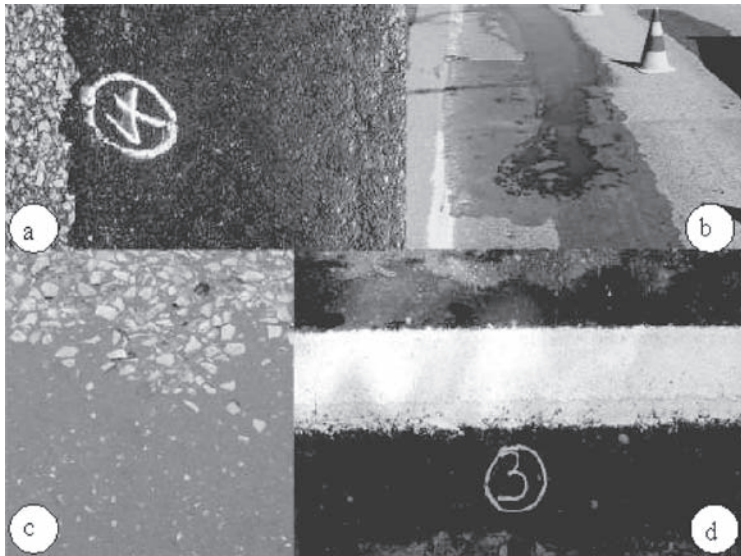
Figure 3. Test sites for gussasphalt patches; (a) on road 140/4, (b) on road 152, (c) on road 140/2 and (d) on road 140/3.
