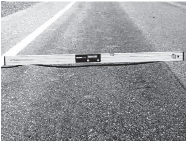
Figure 1. Asphalt pavement rutting due to heavy loads.
