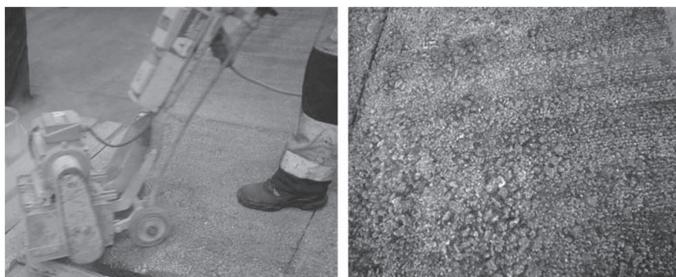
Figure 4. Left: Fine milling device, Right: Surface of base layer after fine milling.
