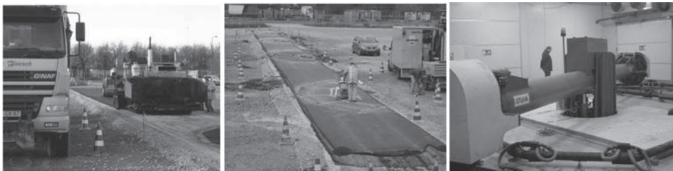
Figure 9. Left to right; test slab construction by using regular road building equipment, retrieval of test slabs, view on STUVA's APT.
