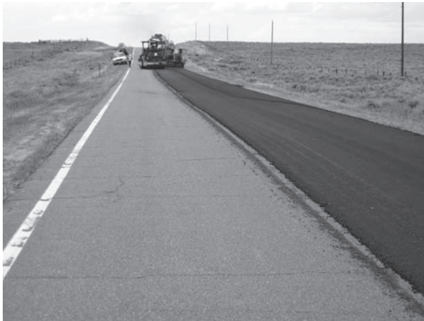
Figure 3. Condition of State Highway 125 in Colorado with transverse cracking on the left lane before CIR on the right line.
