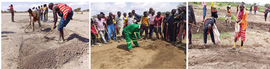
Fig. 3.13 Restoration activities in Mortikanju: bund construction (L), and reseeded (M and R) (Photos: MWCT 2021)
