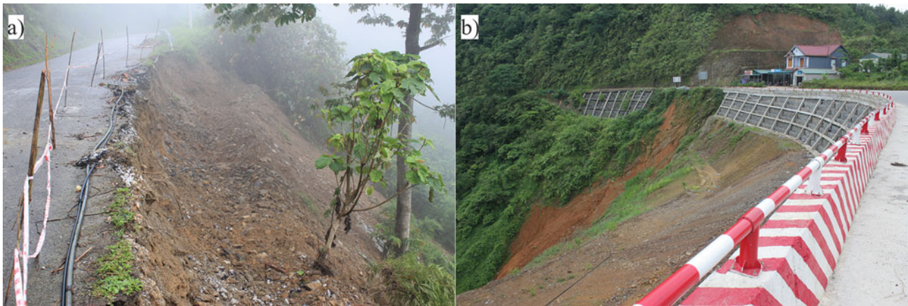
Fig. 2 Landslides at the national highway 34 km 192 + 500 (a), and at Km 200 + 300 (b). Photo by T. K. Nguyen
