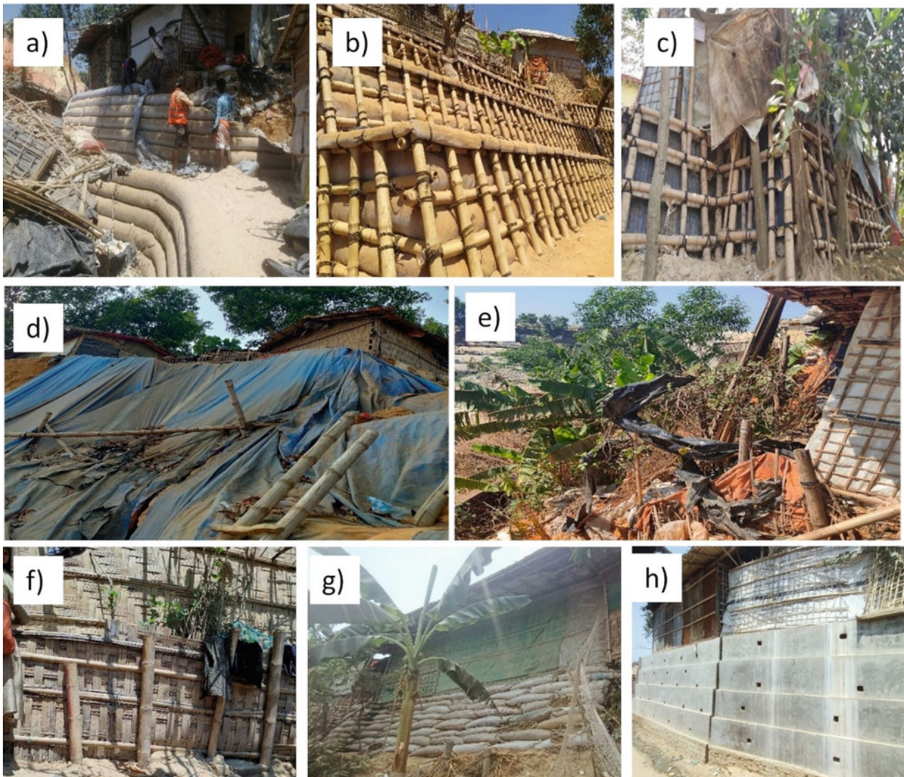
Fig. 2 Different types of structural mitigation measures exist on the slopes of the camp area (a) terrace of geotextile tubes, (b) Terrace of geotextile tubes supported by bamboo fences, (c) terrace of tin sheets
