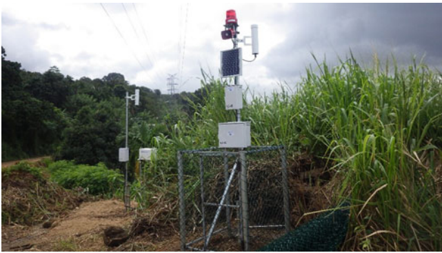
Fig. A.42 Compact alarm device to alert local people to landslide risk
