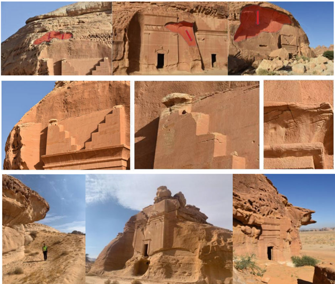
Fig. 10 Example of the main instability processes affecting the different tombs in Hegra: upper sequence of photos stands for rock slide and free fall; middle sequence is reporting small cracks, fractures and
