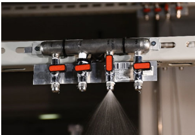
Fig. 3 Photo of one branch with four axial-flow full-cone spraying nozzles
