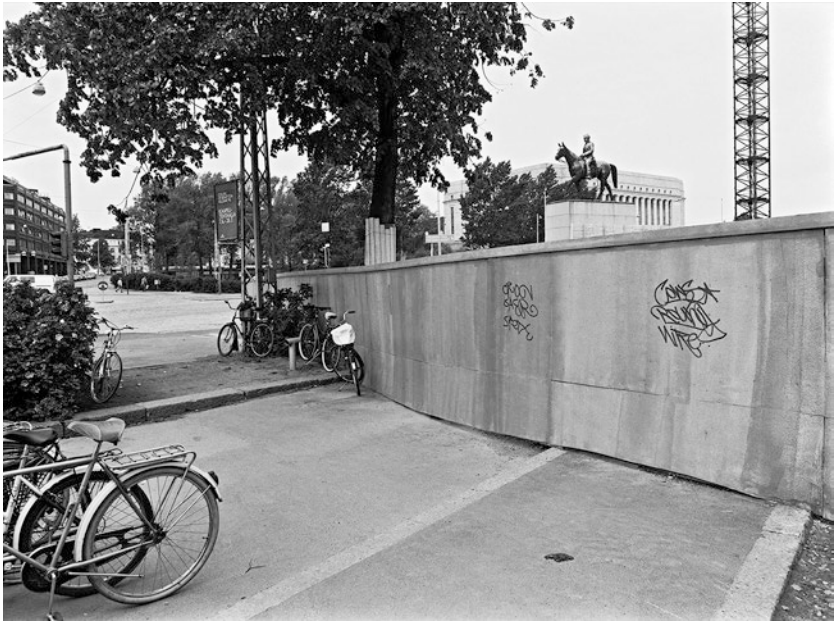
Fig. 14.1 The construction site of Kiasma, the Museum of Contemporary Art in Helsinki, 1996. (Photo: Jan Alanco, Helsinki City Museum)
