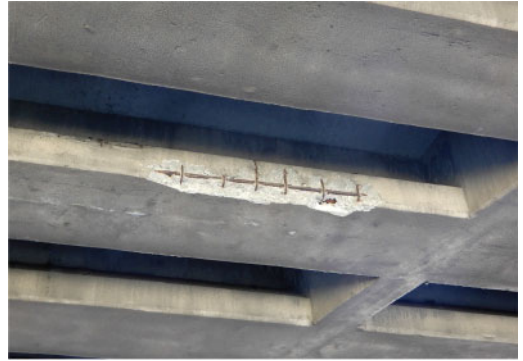
Figure 3. Corrosion damage of the reinforcement in the central bridge girders.
