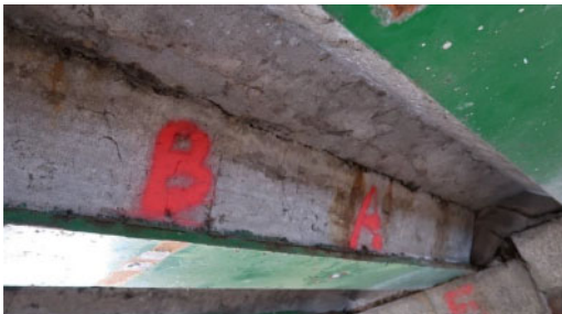
Figure 2. Concrete cracks located at the voute.
