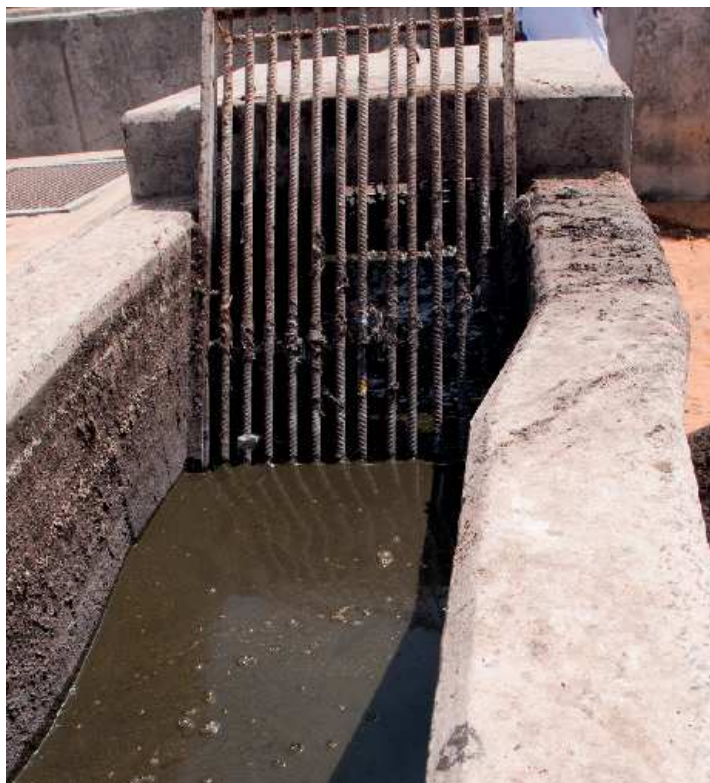
Figure 3.6 Bar screen at Niayes faecal sludge treatment plant, Dakar, Senegal (photo: Linda Strande).
