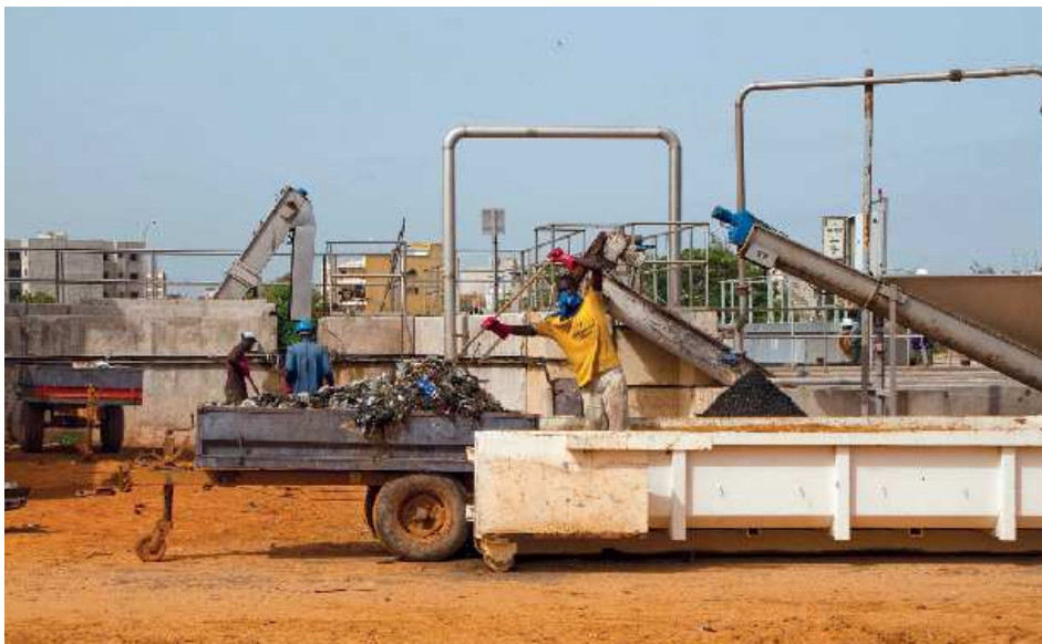
Figure 11.1 Maintenance worker cleans mechanical screens, a critical activity to be performed each shift to keep the system operational, Dakar, Senegal (photo: Linda Strande).
