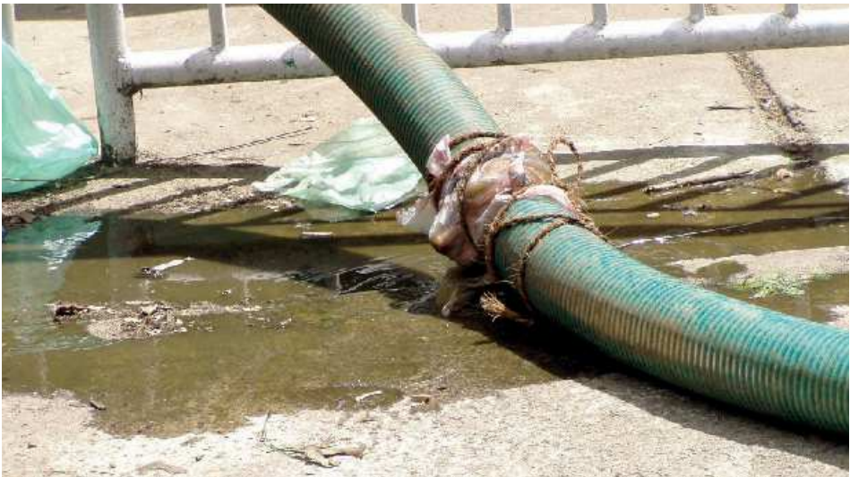
Figure 4.4 Hoses and fittings require frequent attention and repairs to keep them functioning properly. This picture illustrates inadequate maintenance, resulting in leaking of FS from the emptying hose (photo: David M. Robbins).
