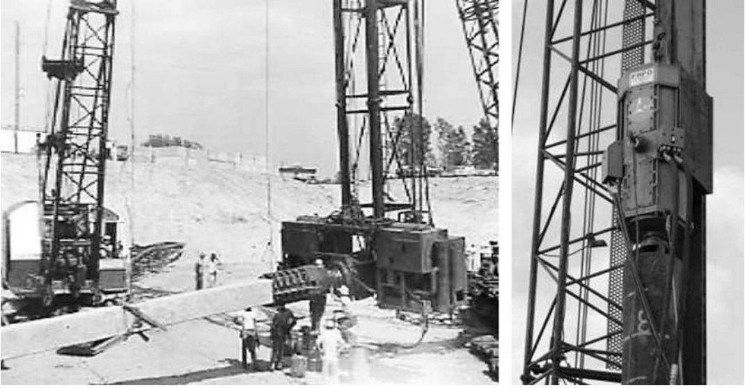
Fig. 5.3 (Left) Job site during preparation to drive a pile using resonant excitation provided by two engines from a Sherman tank. The engines provided counterrotation of eccentric masses (see Fig. 5.4) that drove the pile at its longitudinal standing wave resonance frequency. (Right) A 140 kW (200 HP) resonant driver, mounted on a 60 cm diameter steel pile, that uses a high-speed hydraulic valve to drive the pile at resonance. (Photographs courtesy of Matthew Janes)
