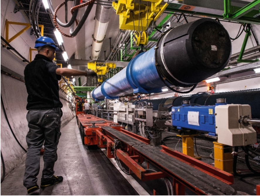
Fig. 4.8 Handling of an LHC dipole magnet with an overhead crane in the LHC tunnel. Copyright CERN, reused with permission
