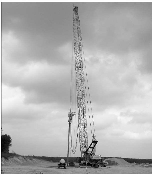
Figure 4.5 Crane-hung dry bottom feed system for deep stone columns (S-Alpha system). (Courtesy of Keller Group plc, London, UK.)
