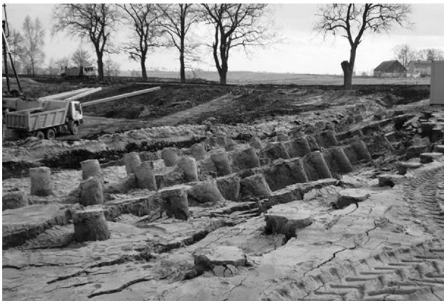
Figure 5.3 Damage to vibro concrete column heads caused by uncontrolled heavy site traffic. (Courtesy of Keller Group plc, London, UK.)
