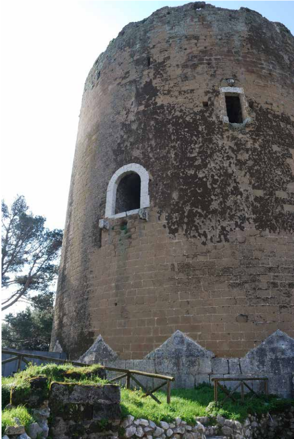
Fig. 5: The 13th-century tower at Casertavecchia (Caserta): the traditional dating depends on the parallelism between the tower travertine basis and the similar architectural feature for those of the gates of Capua, which were built by Frederick II (© Nicola Busino).
