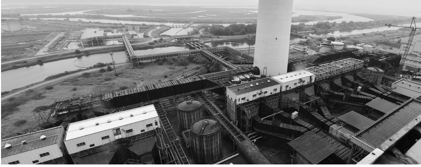
FIGURE 14.17 Intricate system of tubes and pipes in the proximity of the chimney. Source: Chiara Geroldi and Gloria Pessina.
