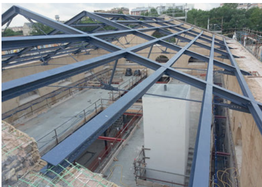
Fig. 8: First phase of the working process for the roof construction, made of steel structures. © Cesare Feiffer.
