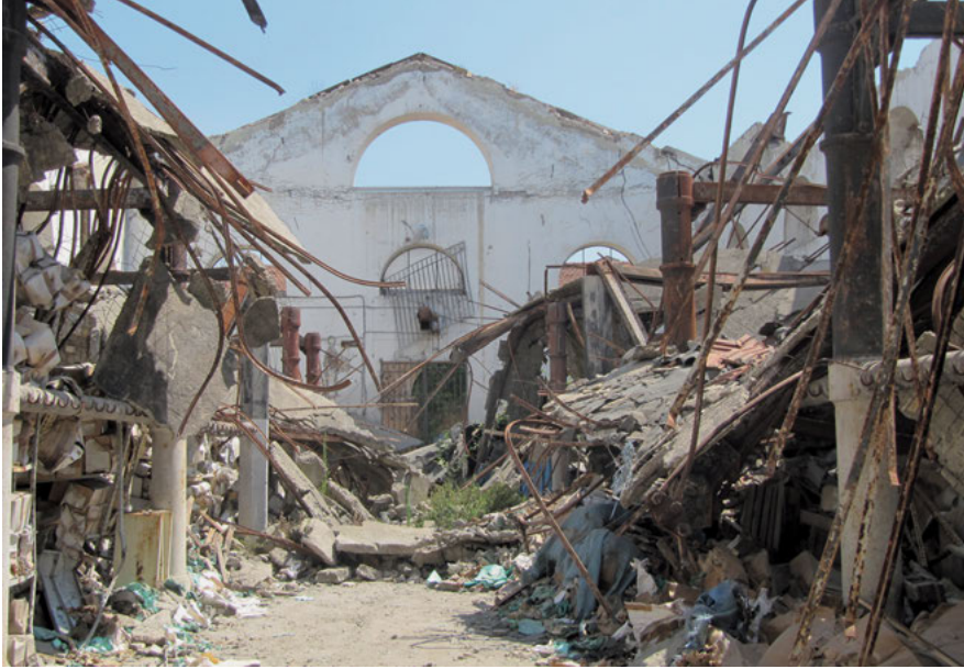
Fig. 5: The Pavilion 9E after the collapse in 2008. © Anna Raimondi.
