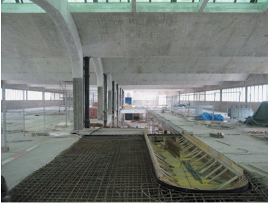
Fig. 8: The central element of the reconstruction work is a cut through the concrete ceiling. © Michael B. Frank.
