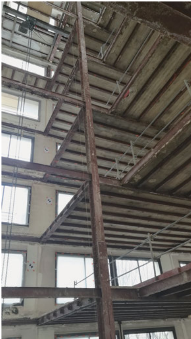
Fig. 3: All interior partitions, finishes, stairs and elevator were removed, and the structure stripped away to its core. © Lia Kiladis architecture.
