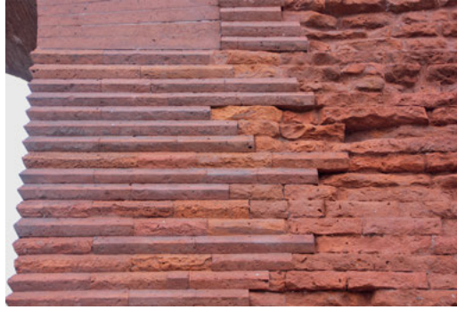
Fig. 3: Turin, main gate of the Porta Palatina, meticulous brickwork on the façade.
