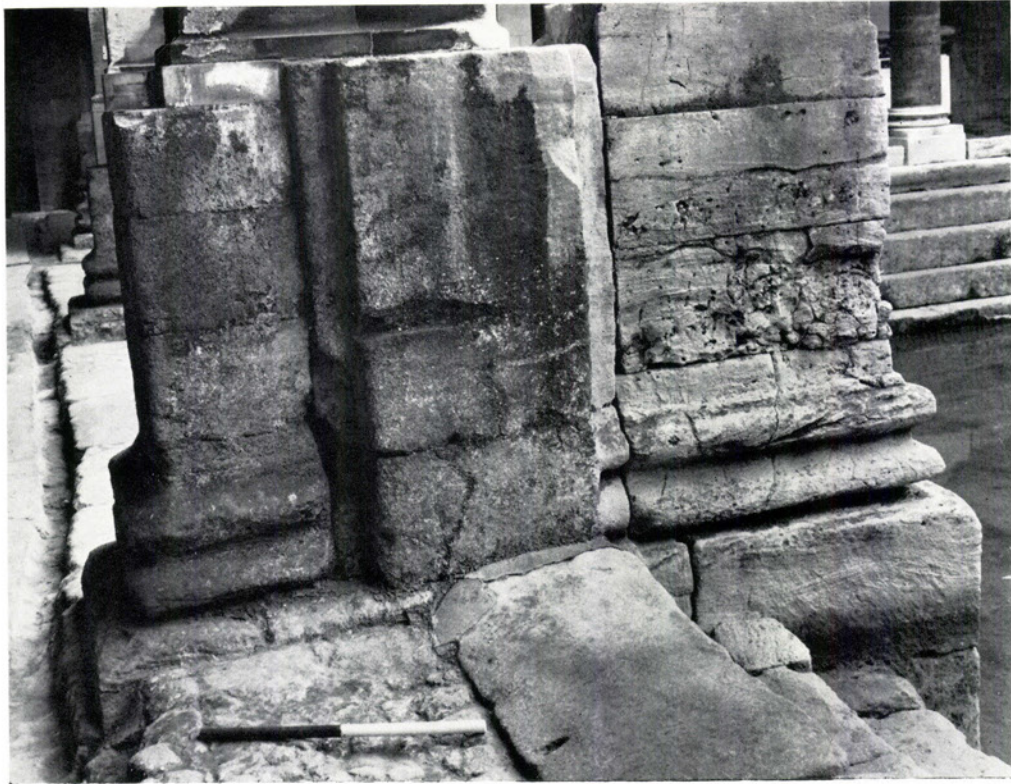
a. The Great Bath: one of the first-period piers on the north side of the bath, showing the additional strengthening piers of the third period (p. 98)
