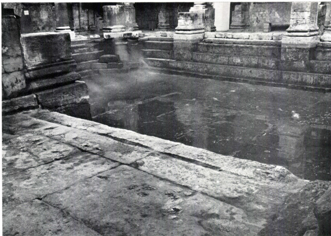
a. The south side of the Great Bath, showing the run-off channels cut into the top step (p. 96)
