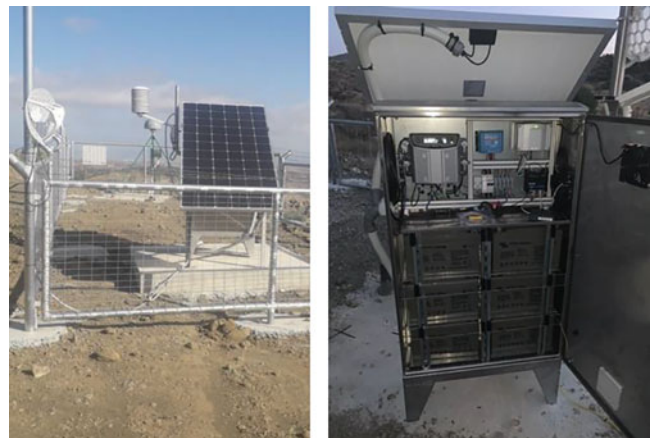
Fig. 6 The integrated enclosure—solar panel configuration used in CyCLOPS permanent and mobile stations
