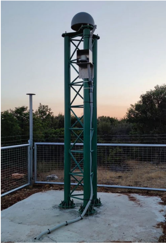
Fig. 4 The stainless steel truss monument type specifically designed for the stability requirements of the CyCLOPS permanent segment
