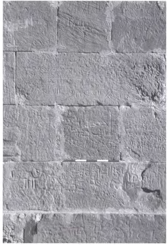
Fig. 8.38. Graffiti on Garamantian structure (UAT 1).
