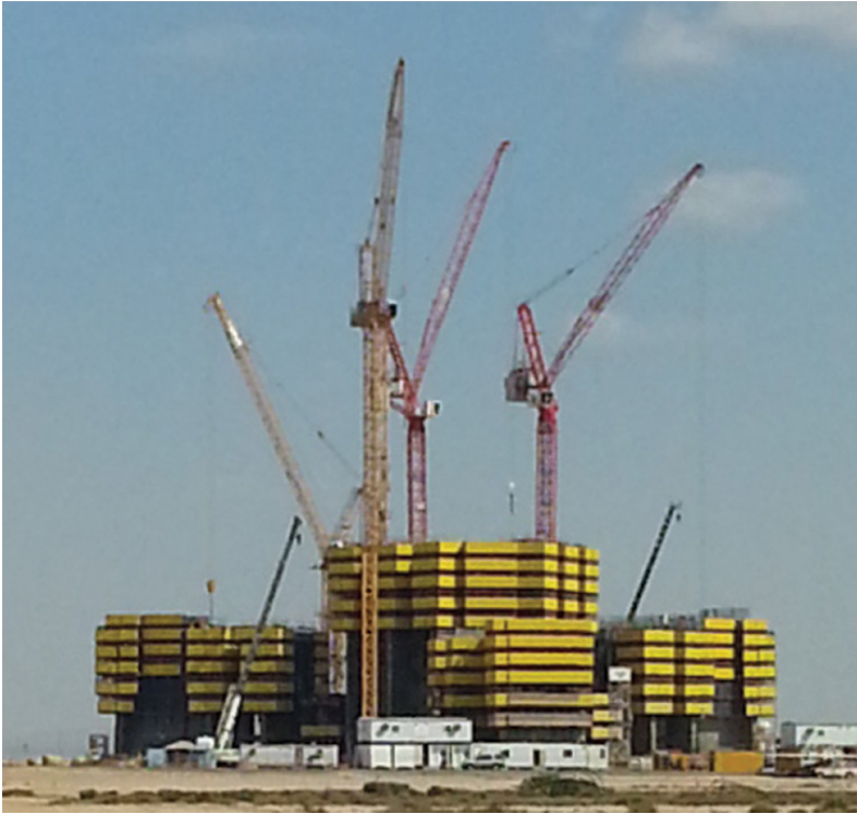
Figure 12.1 Construction of the Kingdom Tower in Jeddah, February 2015. Source: Ammar Shaker (CC BY-SA 4.0).
