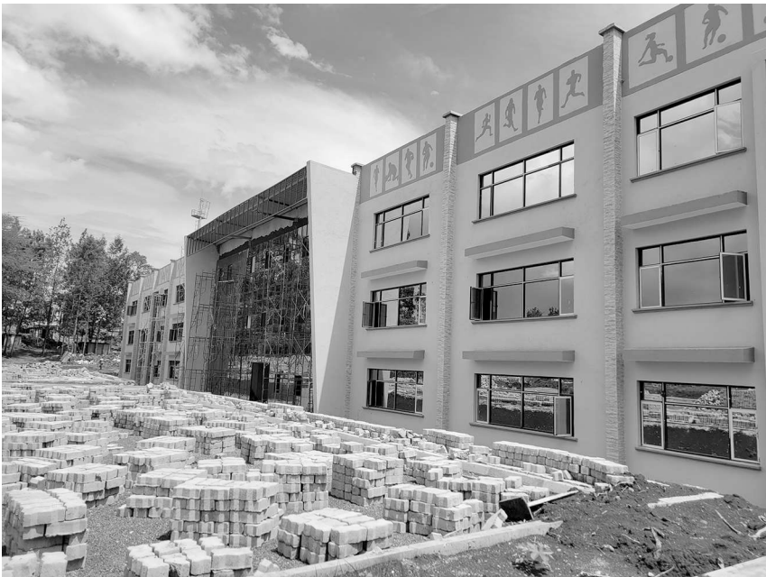
FIGURE 13.2 Front façade of Kirigiti Stadium in Kiambu County, under construction in January 2022
