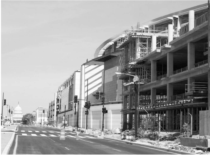
FIGURE 10.2 Nationals Park, under construction in 2007. (Photo by Aude is licensed under CC BY-SA 3.0)
