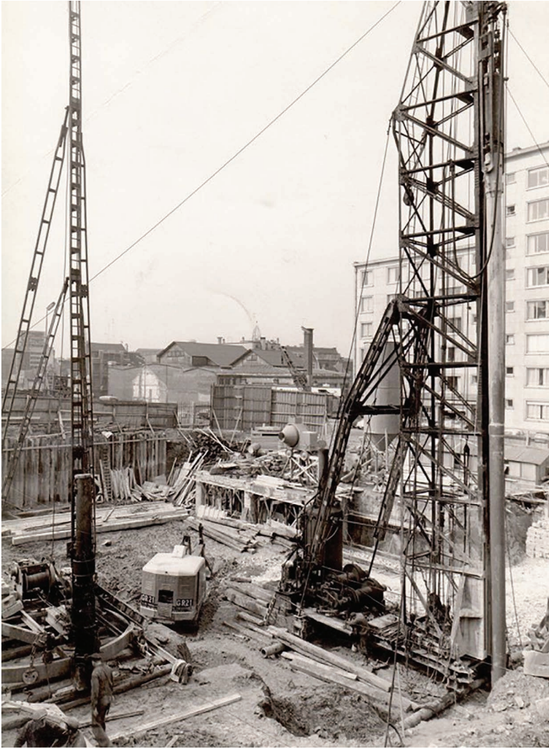
Figure 2.2.5 Execution of Vibro cast in situ piles for the foundations of a Boulevard Pacheco office building (Brussels) in 1961.
