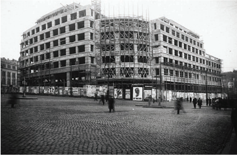
Figure 2.2.16 The Shell building under construction at the corner of the rue Ravenstein and the rue Cantersteen, Brussels, around 1932. Architects, Alexis Dumont and Marcel Van Goethem.
