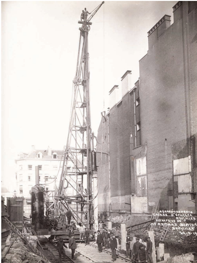
Figure 2.2.3 Driving prefabricated reinforced concrete piles for the foundations of the extension of the Caisse d'Epargne savings bank in Brussels (photograph dated 24 September 1912).
