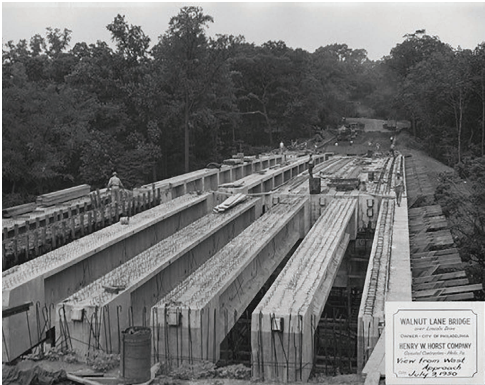
Figure 2.2.19 The Walnut Lane Bridge over the Lincoln Drive in Philadelphia under construction.
