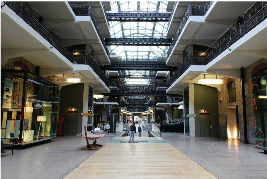
Figure 1.6.6 Cantilever balconies in reinforced concrete at the Royal Tour & Taxis warehouse (1903–1907) in Brussels.
