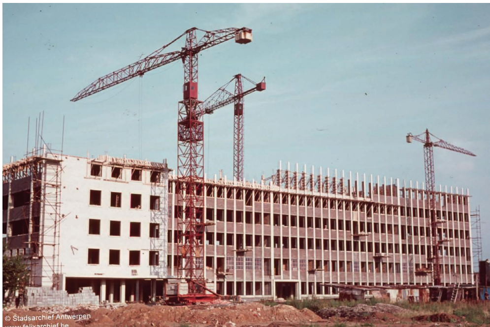
Figure 2.4.10 Construction of St Erasmus Hospital in the later Antwerp district of Borgerhout by contractor Verachttert, 1966.
