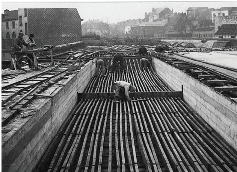
Figure 2.2.11 Laying the Sandwich cables for the railway bridge deck over the rue du Miroir (Brussels) in 1943 (or 1944).
