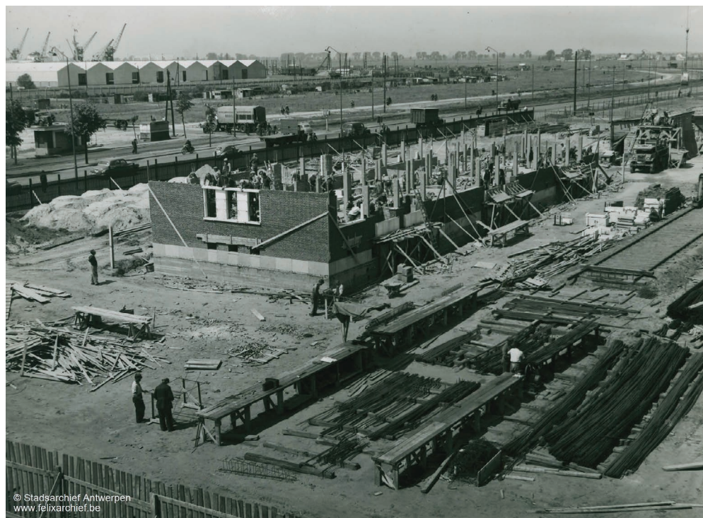
Figure 2.4.7 Construction of Darsen XII social housing blocks at Antwerp Luchtbal by contractor Verachttert, circa 1955.
