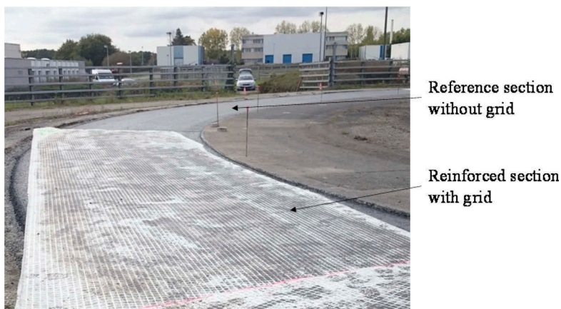
Figure 1. Full-scale pavement sections with and without glass fiber grid reinforcement before application of the overlay during the construction.
