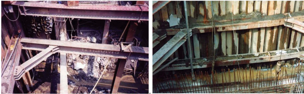
Figure 1. Groundwater flooding on excavation finish surface.
