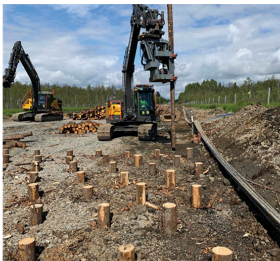
Figure 4. Pile driving using an excavator with a grip claw. The piles in the foreground have been trimmed down to the pile cut-off level. Photo: Hjalmar Törnqvist, AFRY.
