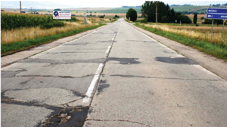
Figure 1. Example of distress of pavement (first class road I/65).
