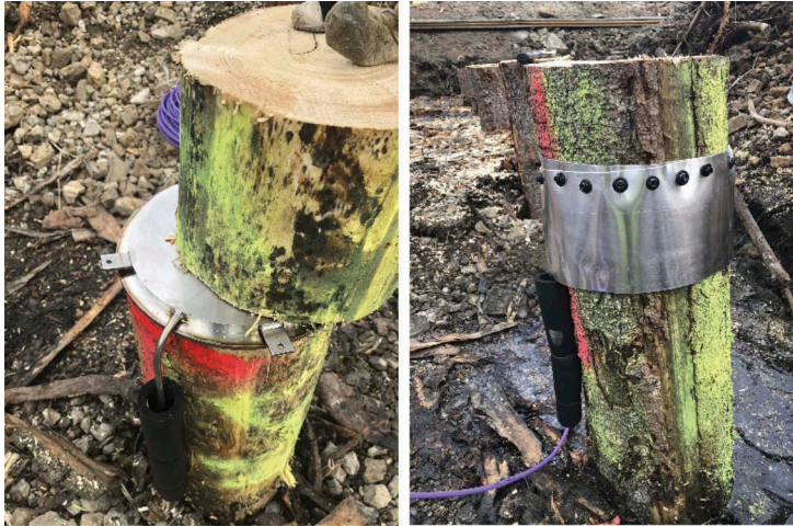
Figure 7. To the left: view of pressure cell installed inside a timber pile. To the right: view of protective aluminium sheet around the pressure cell inside the pile.
