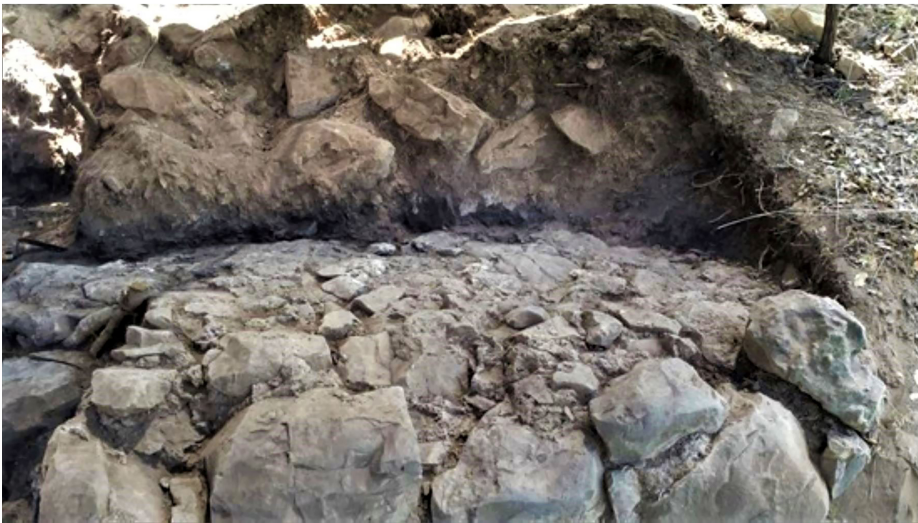
Fig. 20: Undermining of the domestic building (a) and the westernmost building (b) (© Adrian Boas and Rabei Khamisy).
