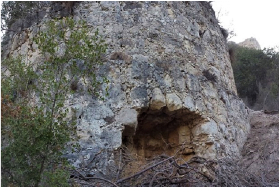
Fig. 19: Undermining of the administrative building (a) and the south-western tower (b) (© Adrian Boas and Rabei Khamisy).
