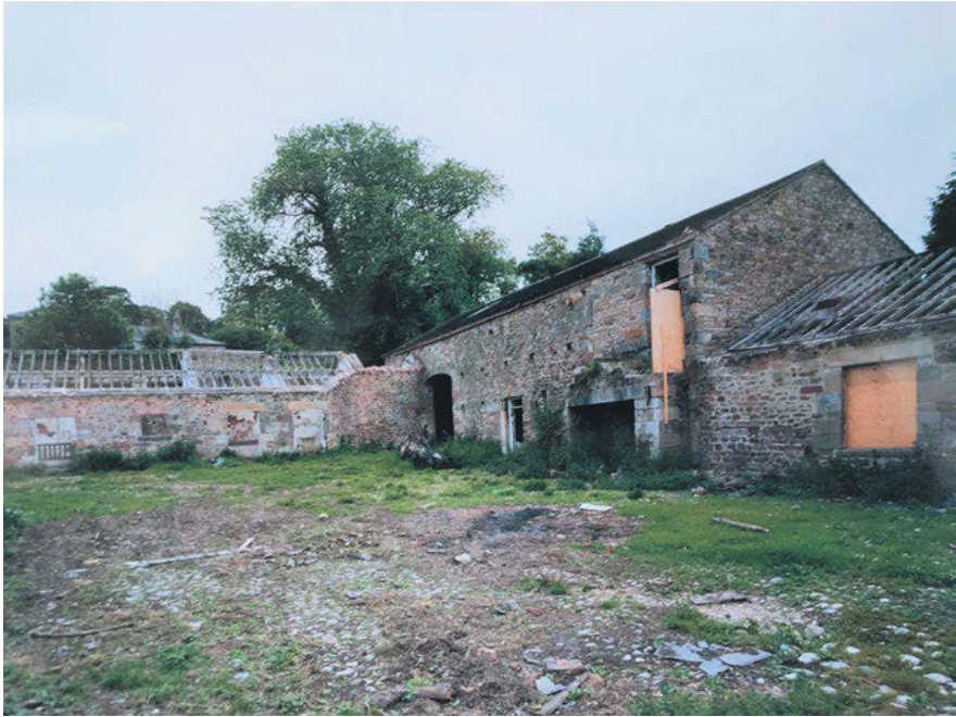
Figure 21.1: Derelict farm buildings before they were converted into dwellings. (Photo by: Gordon Walker).
