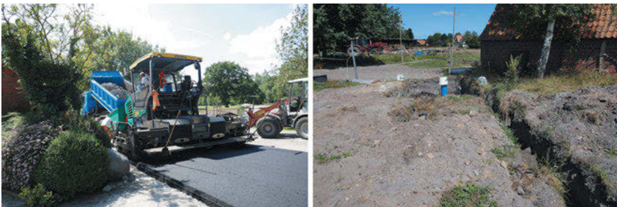
Figure 34.2: Paving the Flax Road (left) and installing the irrigation system (right) (Photos by: Werner Krauß).
