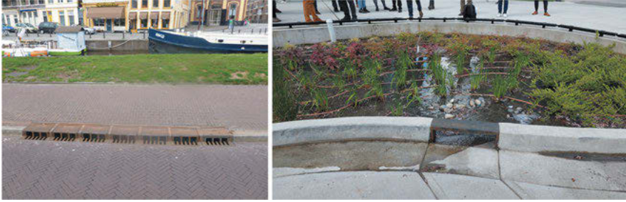
Figure 32.1: From grey underground infrastructure (left) to grey-green surface infrastructure (right). (Photos by: Floris Boogaard).
