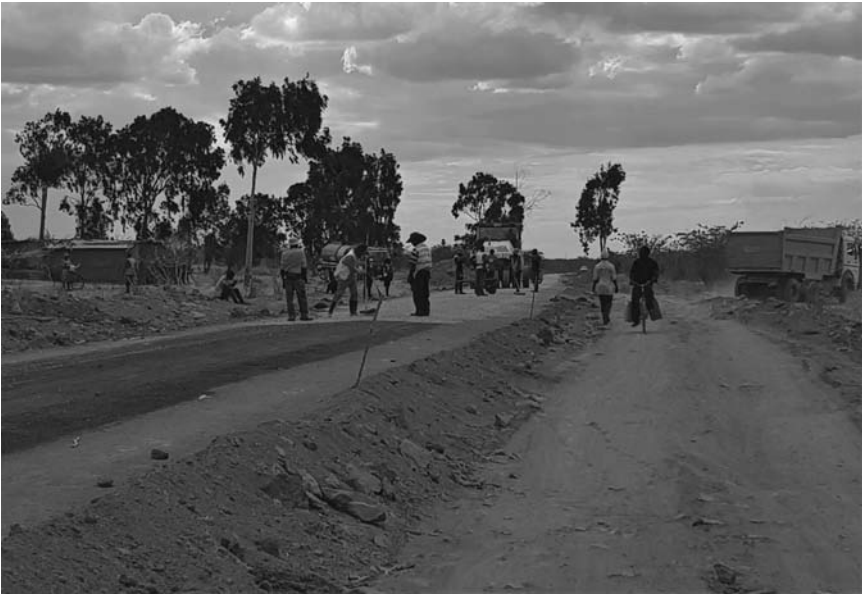
Figure 15.4 Construction of the metalled surface of the all-weather road between Ilambilole and Kising'a, November 2017.
