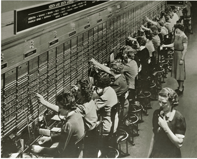
FIGURE 2.1 An example of circuit switching: telephone operators at “Central” using a plug board to connect phone calls.
