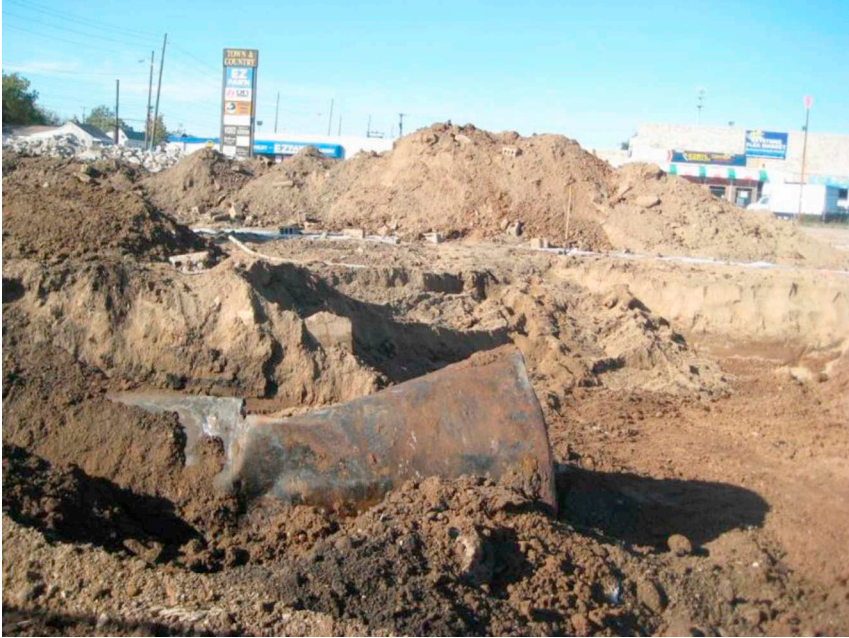
FIGURE 13.1 Underground storage tanks being excavated by the EPA in 2012 in the first phase of mitigation at the Tuchman Cleaners site, Indianapolis, IN (Photo: Environmental Protection Agency).
