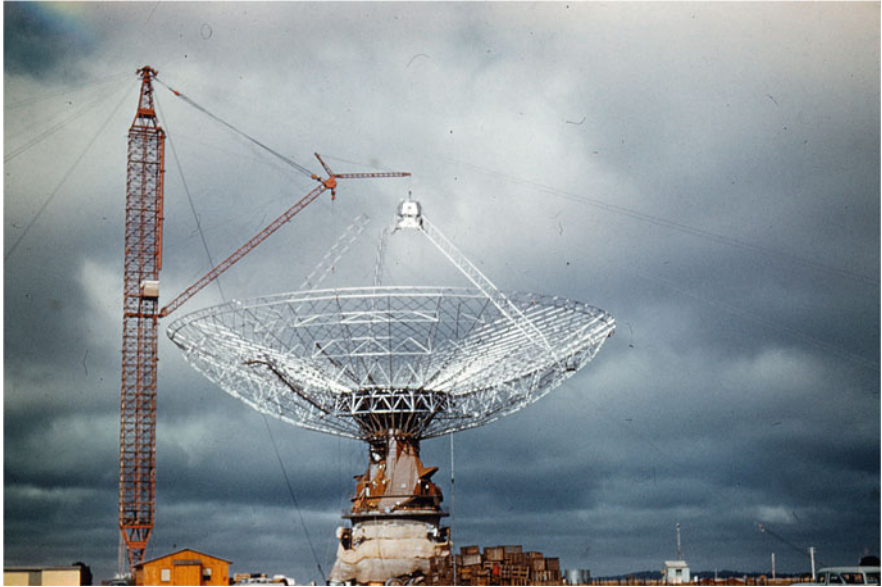
Fig. 32.1 In June 1961, the tripod was positioned with the aerial cabin mounted. This image, on a stormy day, from the Austie Helm collection (via his son Denis Helm and grandson Scott) shows the final moments of the lift. Note the man on the right most feed leg of the tripod. The erection crane was used by MAN for the construction of the telescope starting in late 1960. Credit: Austie Helm Collection, all rights reserved
