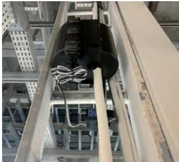
Figure 20. Device installed at Pimental hydraulic power plant in Brazil.
