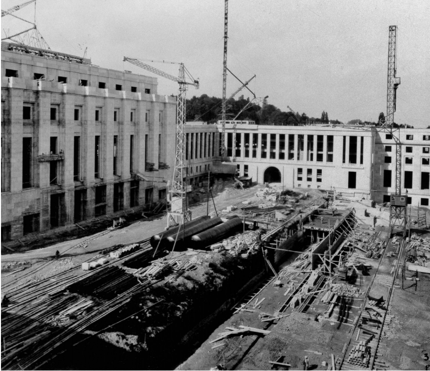
Fig. 12. The Palace of the Nations under construction, 3 October 1933. United Nations Archives at Geneva.
