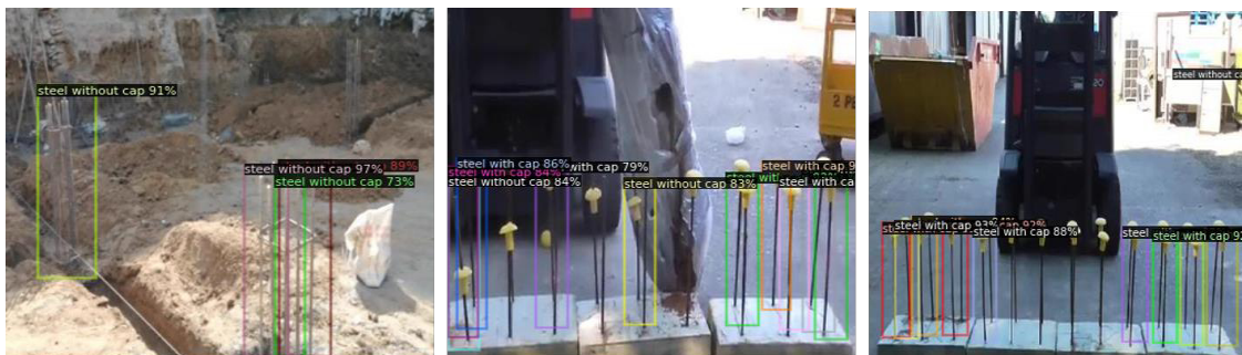
Figure 9: Example of protruding reinforcing steel for Monitoring Work Finish of Certain Level
