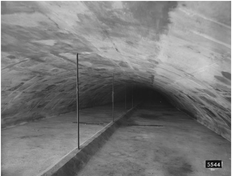
Top : blower air duct, New York land ventilation building; bottom : exhaust air duct, north tunnel
