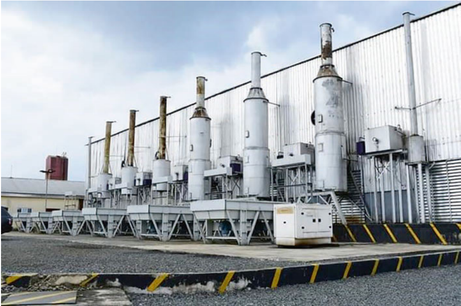
Fig. 8.2 The Calabar Power Plant in 2021
