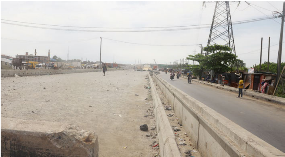
Fig. 9.3 The state of much of the Lagos-Badagry Express Road ten years into the project
