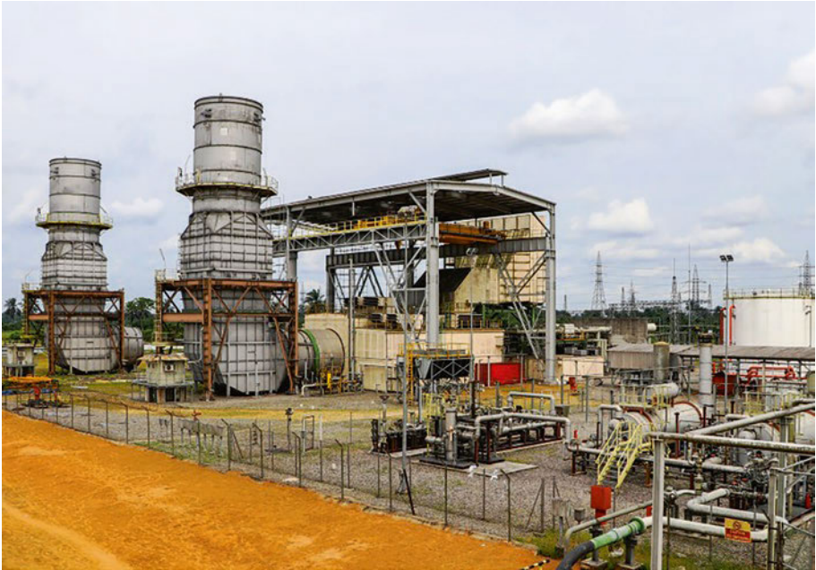
Fig. 4.10 Omoku Power Plant
