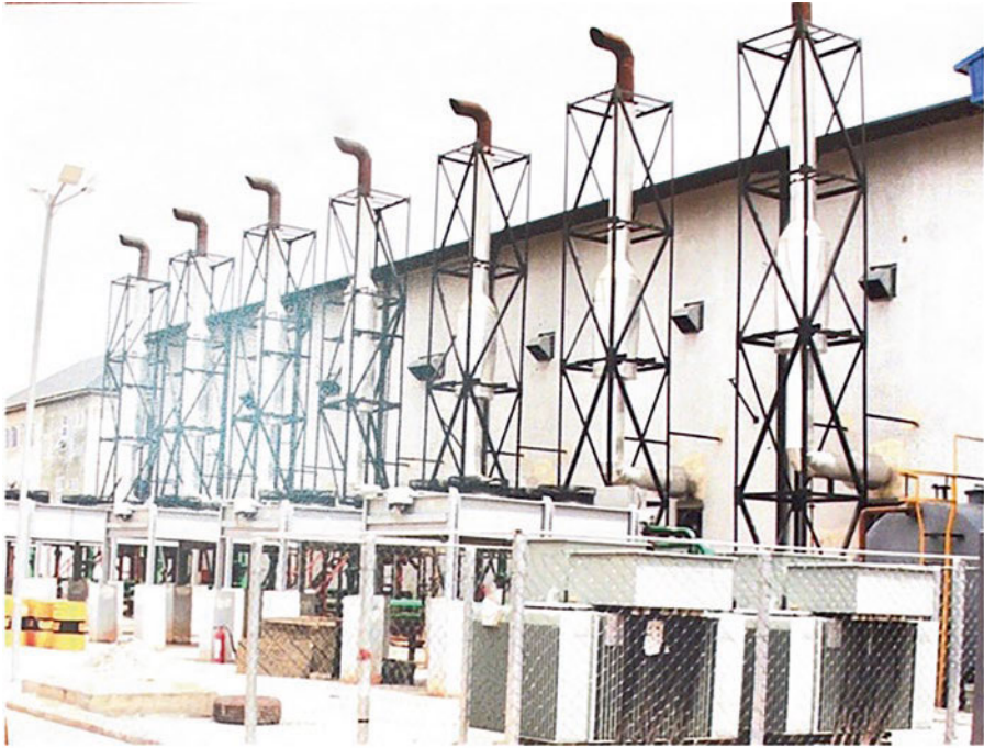
Fig. 4.8 Delta State Oghareki Power Plant
