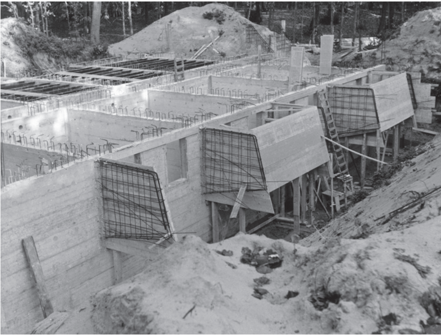
5: The nitrate vaults at Overveen under construction (Collection EYE Film Institute Netherlands)
